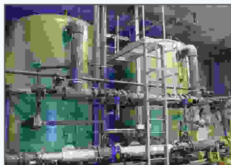
Environmental protection equipment
